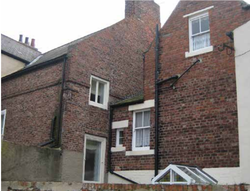
VIEW OF THE REAR AND SOUTH WEST SIDE ELEVATION OF THE MAIN GEORGIAN TOWNHOUSE AND ITS ABUTMENT WITH RED HOUSE
